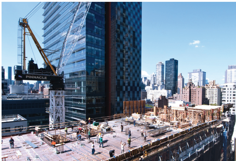
The superstructure of the new 18-story Medical Research Building is now approximately half complete.
